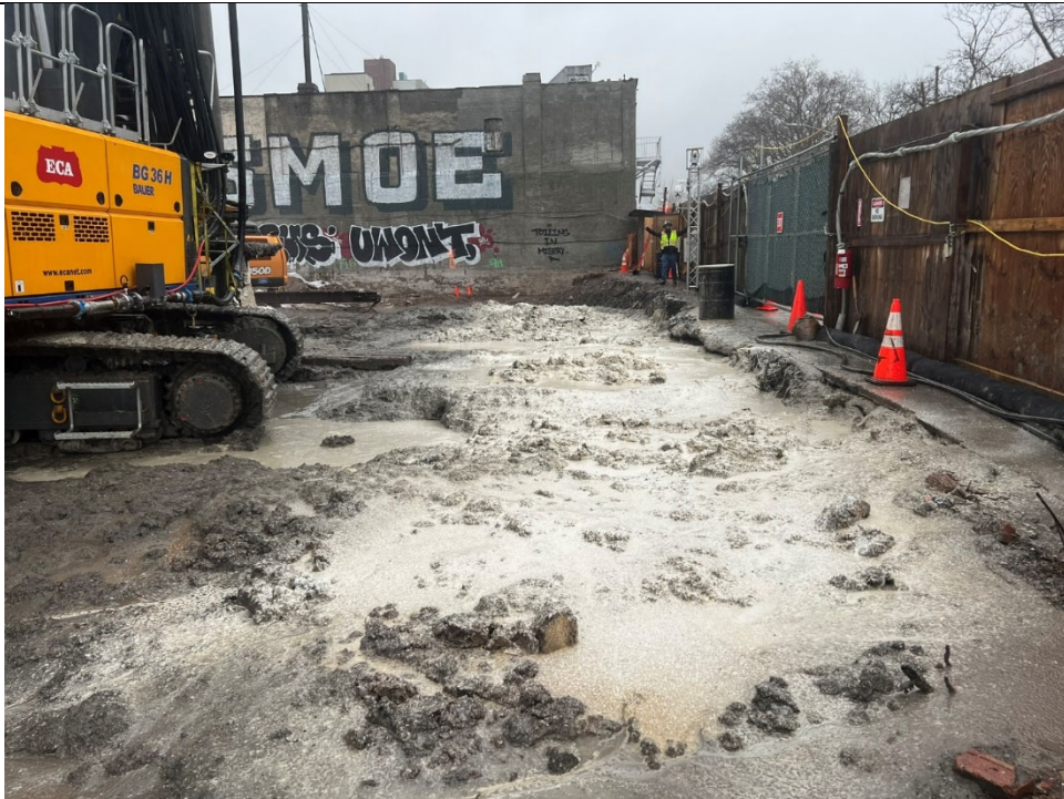
Photo 4- Representative photo of the work area covered with ATMOS foam at the end of the day.
