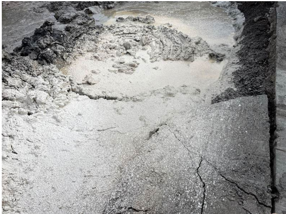
Photo 4- Representative photo of the work area covered with ATMOS foam at the end of the days activities.
