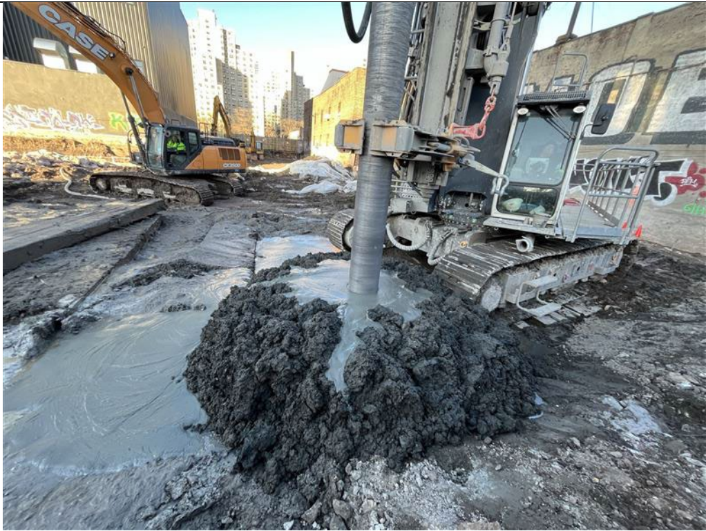
Photo 2- Representative photo of swell from ISS column installation.
