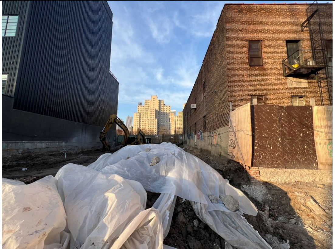
Photo 4- Representative photo of a swell stockpile covered at the end of the day in poly.
