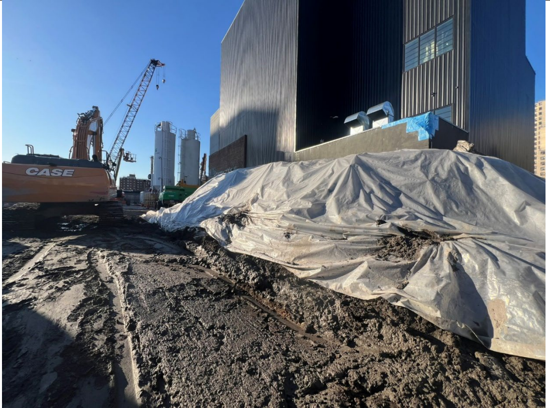
Photo 3- Representative photo of stockpiled swell material covered at the end of the day in poly.
