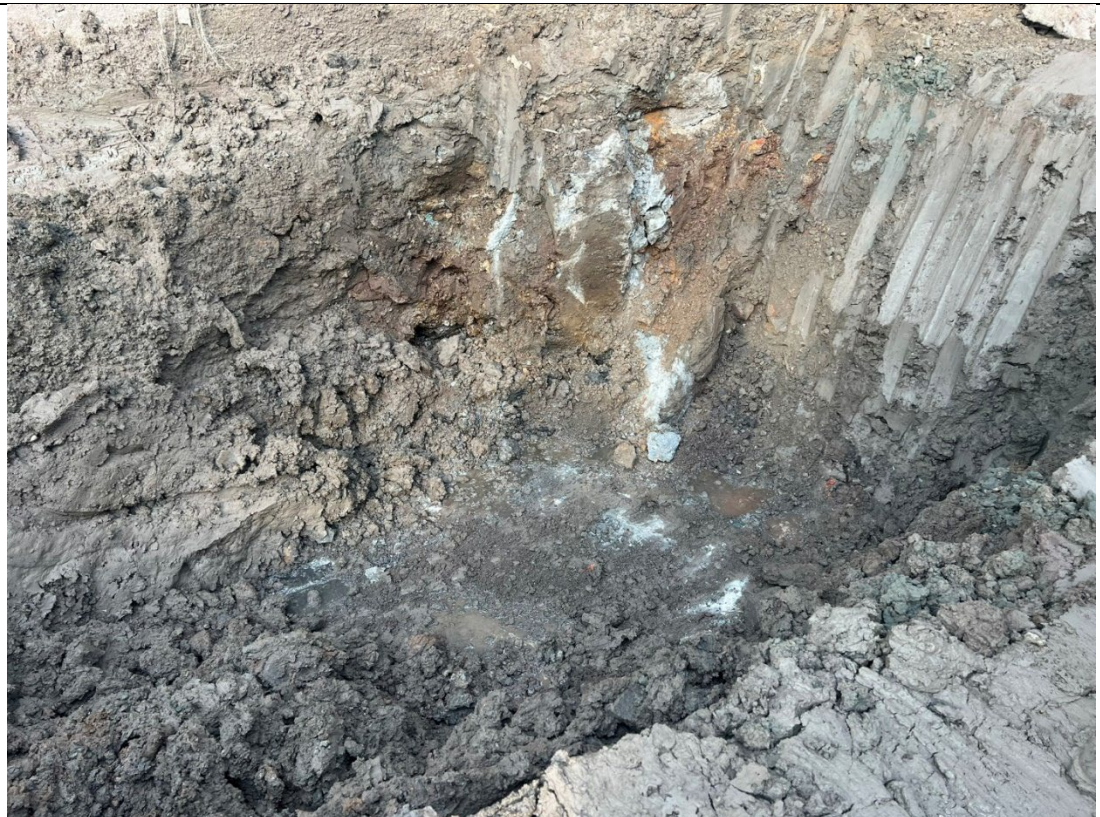
Photo 4- Representative photo of a concrete obstruction found 10' below sidewalk grade.
