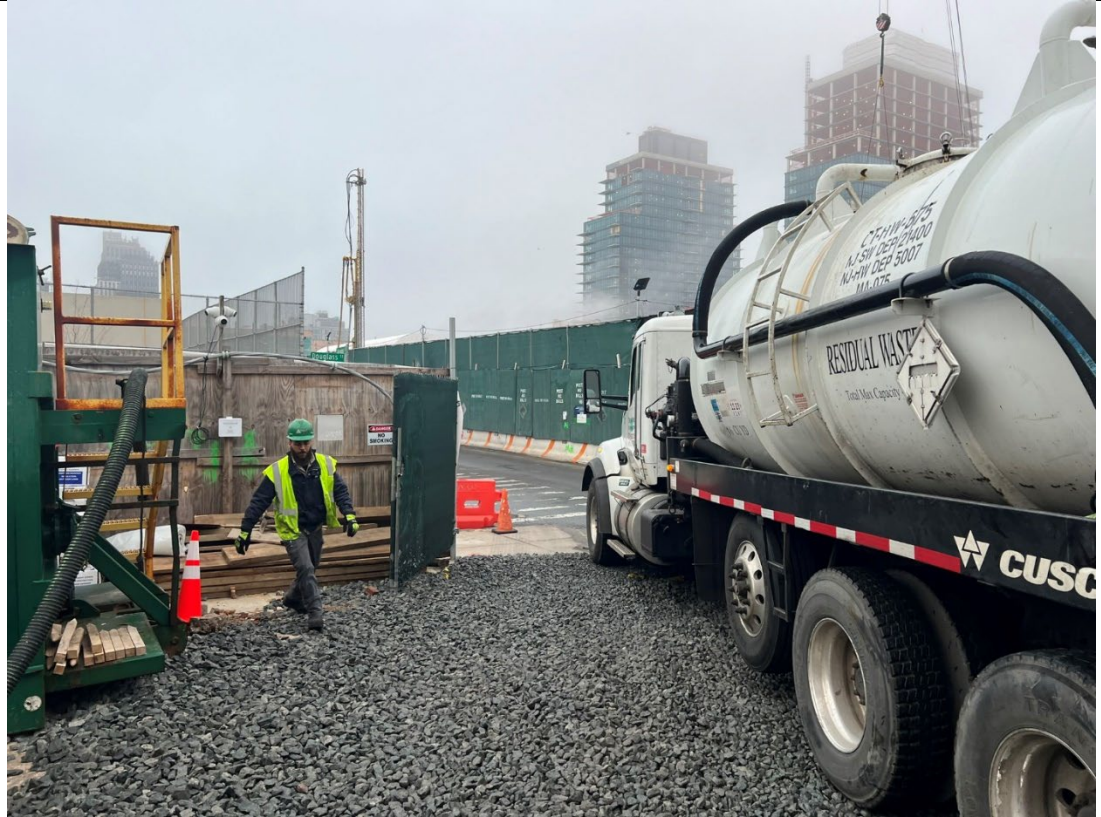
Photo 1- Representative photo of a pump truck removing sampled liquid from the frac tank.
