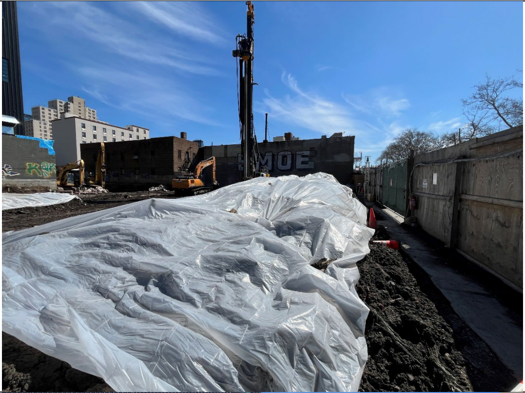
Photo 5- Representative photo of stockpiled swell material covered at the end of day.
