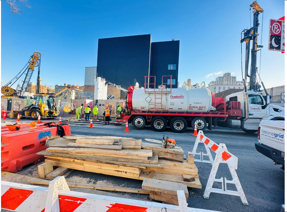
Photo 1- Representative photo of national grid and clean harbor working on side along site at Douglass Street.
