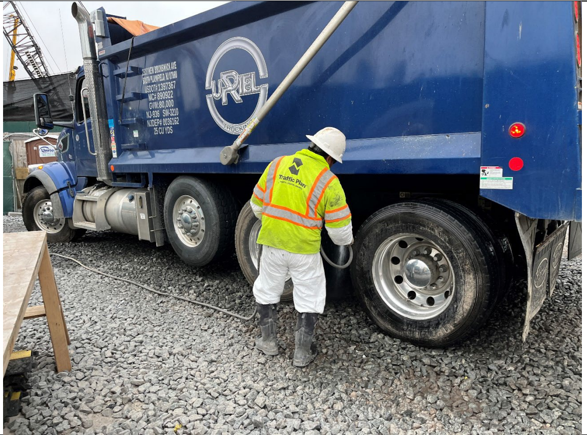
Photo 3- Representative photo of tires being washed over track pad prior to truck exiting the Site.
