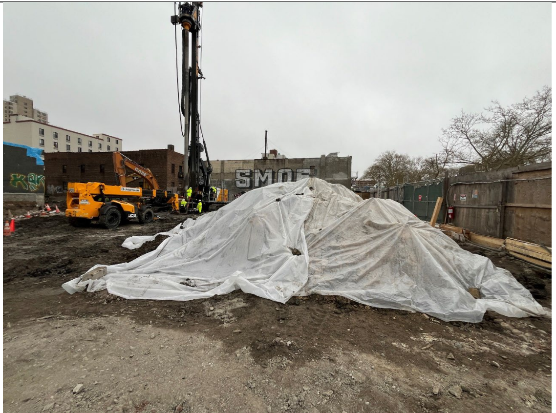
Photo 5- Representative photo of the swell stockpile being covered and secured at the end of the day in poly.
