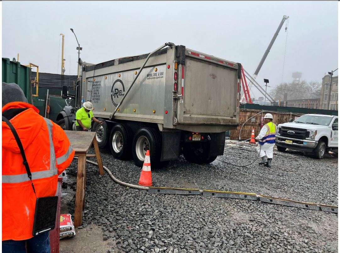
Photo 5- Representative photo of truck tires being cleaned before exiting site over track pad.
