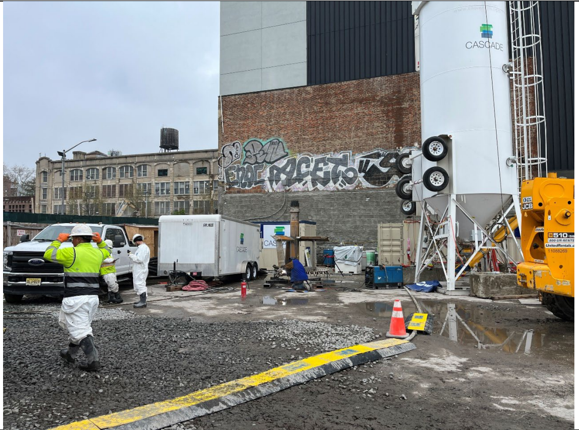
Photo 3- Representative photo of auger maintenance.
