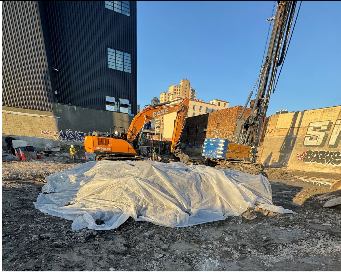
Photo 5- Representative photo of the swell stockpiled securely covered at the end of site activities.
