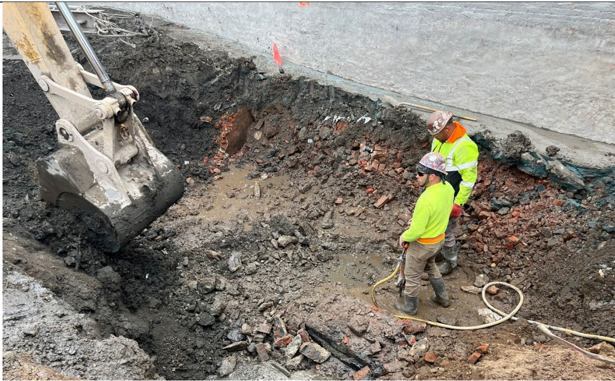
Photo 4- Representative photo of Concrete Courses removing obstructions in the southeast corner of the Site.
