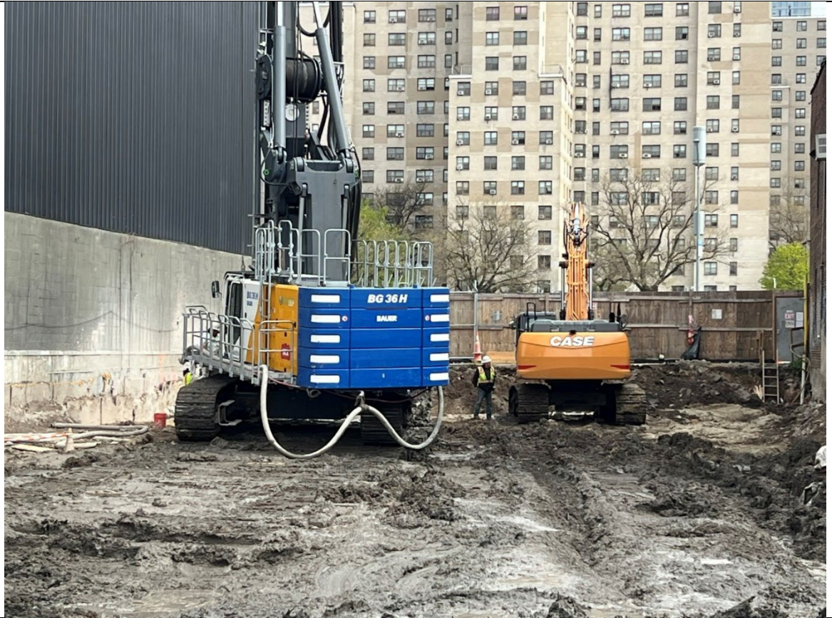
Photo 5- Representative photo of Cascade moving to the northern portion of the Site for ISS column installation.
