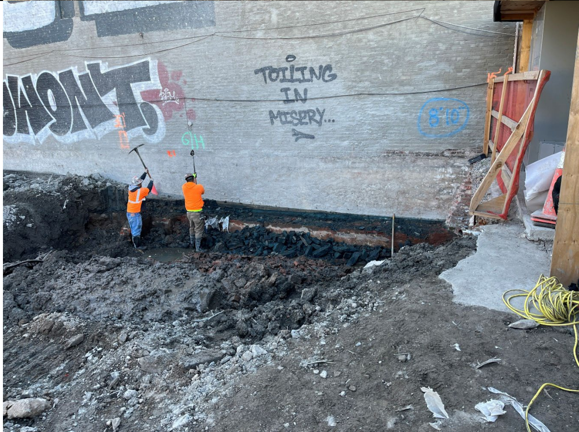
Photo 4- Representative photo of Concrete Courses removing obstructions in the southeast corner of the Site.
