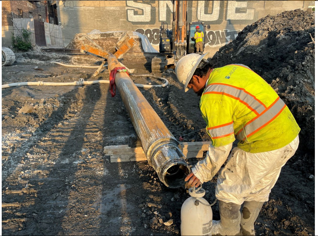
Photo 2- Representative photo of kelly bar repairs.
