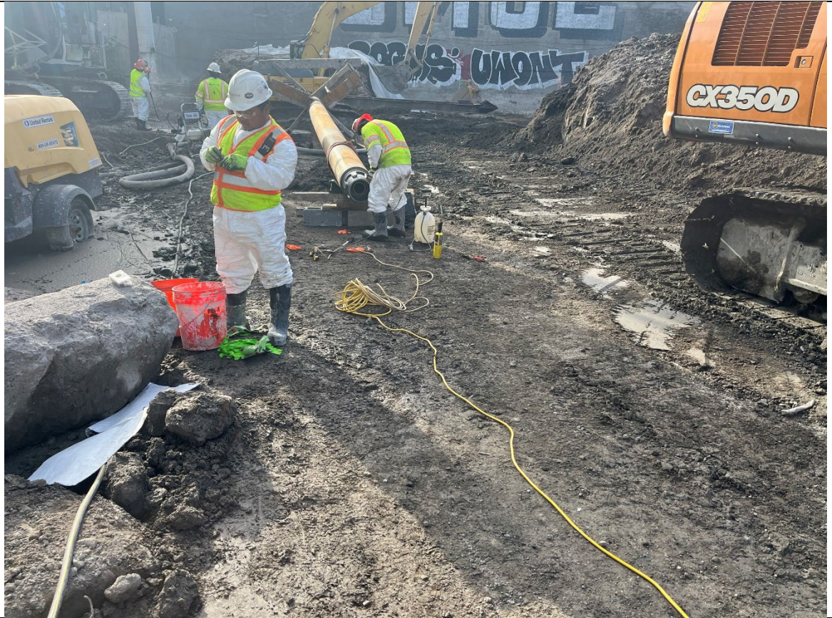
Photo 3- Representative photo of kelly bar repairs.
