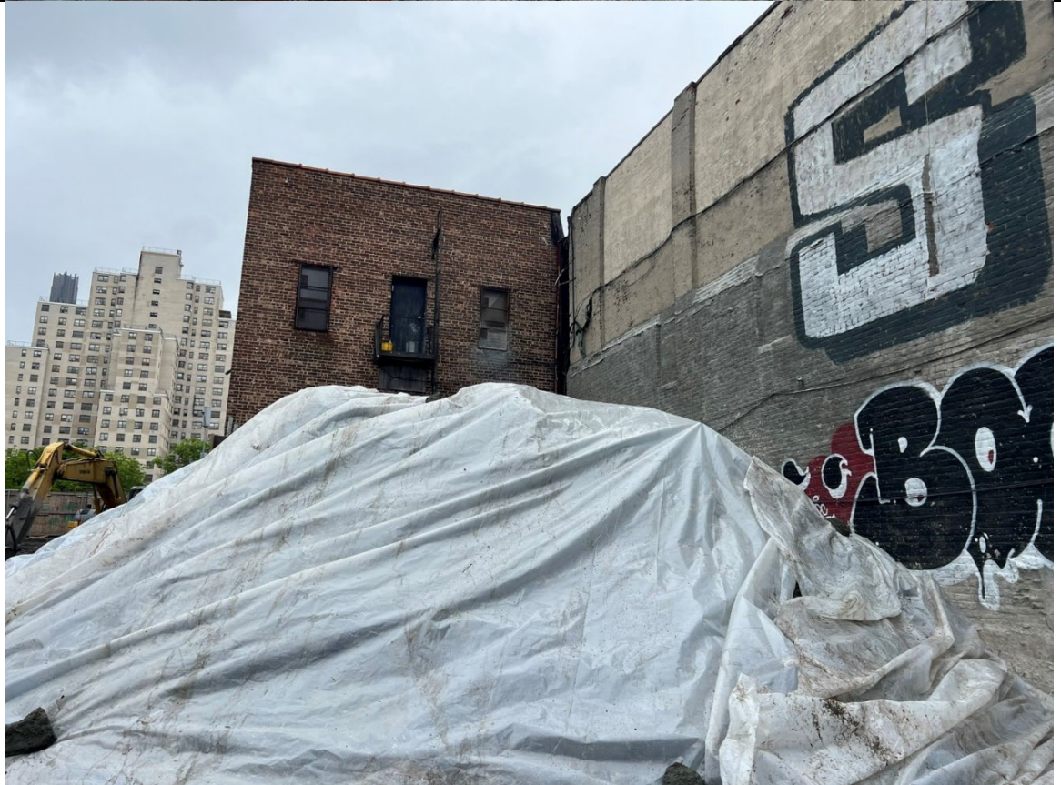
Photo 4- Representative photo of swell stockpile securely covered at the end of the day.
