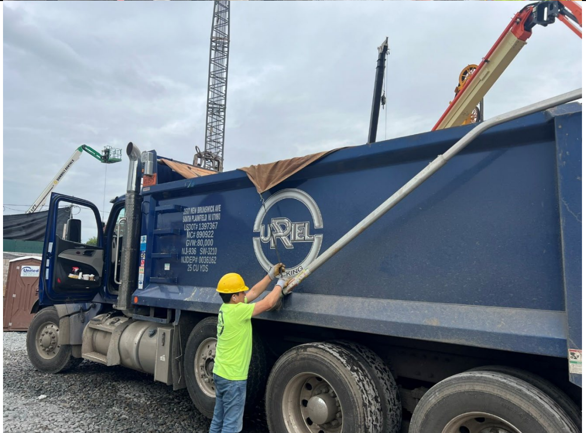
Photo 2- Representative photo of straps being used to secure the sides of the tarp prior to the truck exiting the Site.
