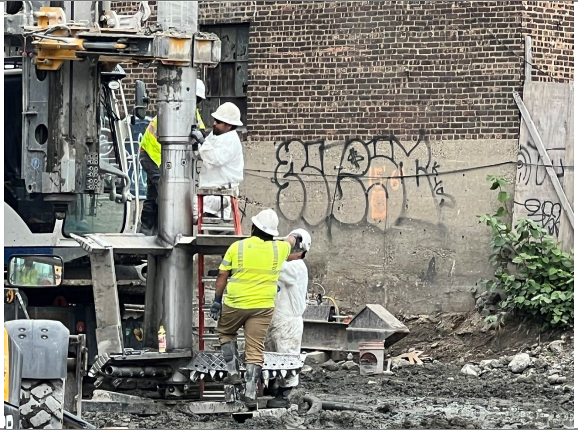
Photo 5- Representative photo of Cascade taking the auger off of the drill rig.
