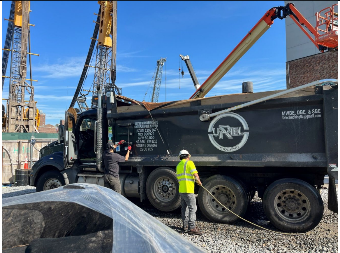
Photo 1- Representative photo of strapped truck cover for swell material prior to exiting the Site.
