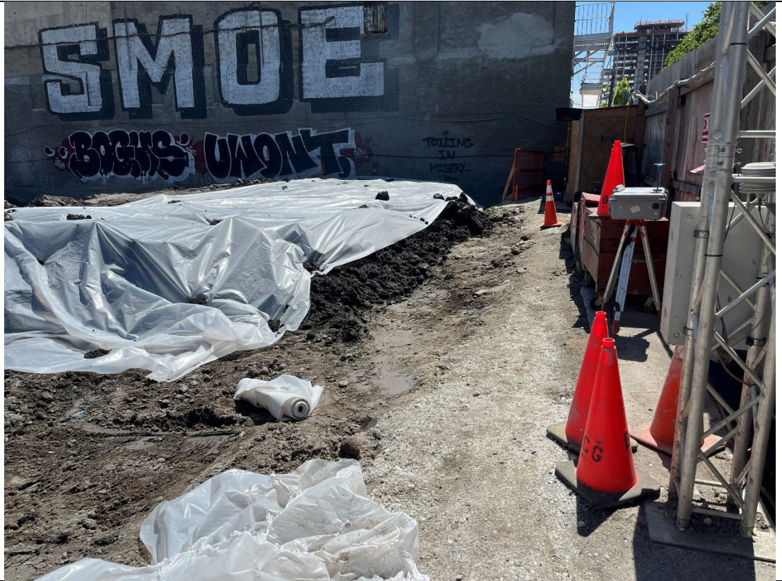
Photo 3- Representative photo of securely covered swell material stockpile at end of day.
