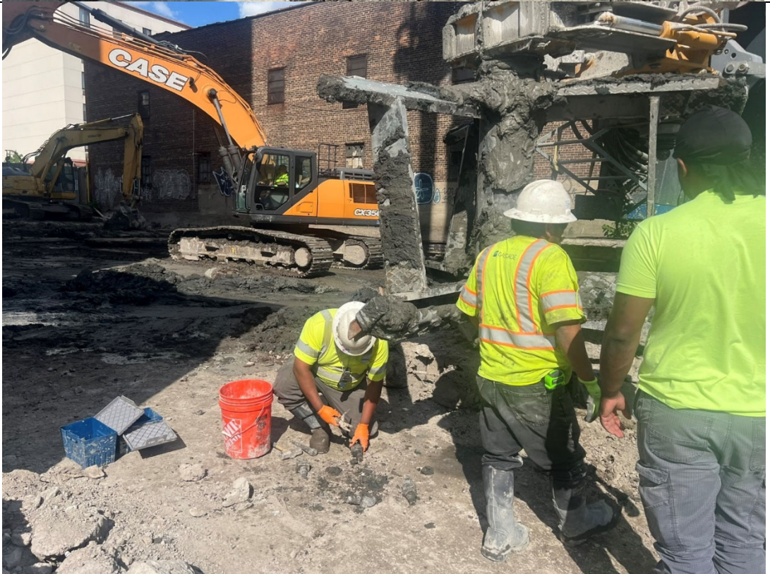
Photo 2- Representative photo of Cascade fixing teeth on auger.
