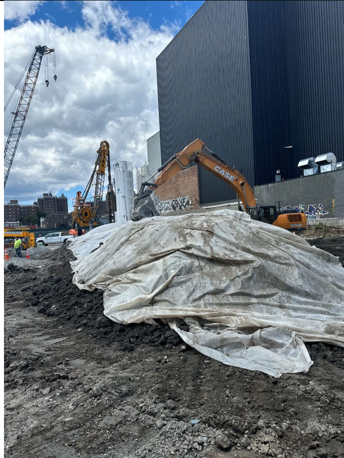
Photo 4- Representative photo of swell stock pile being covered with poly at the end of the day.
