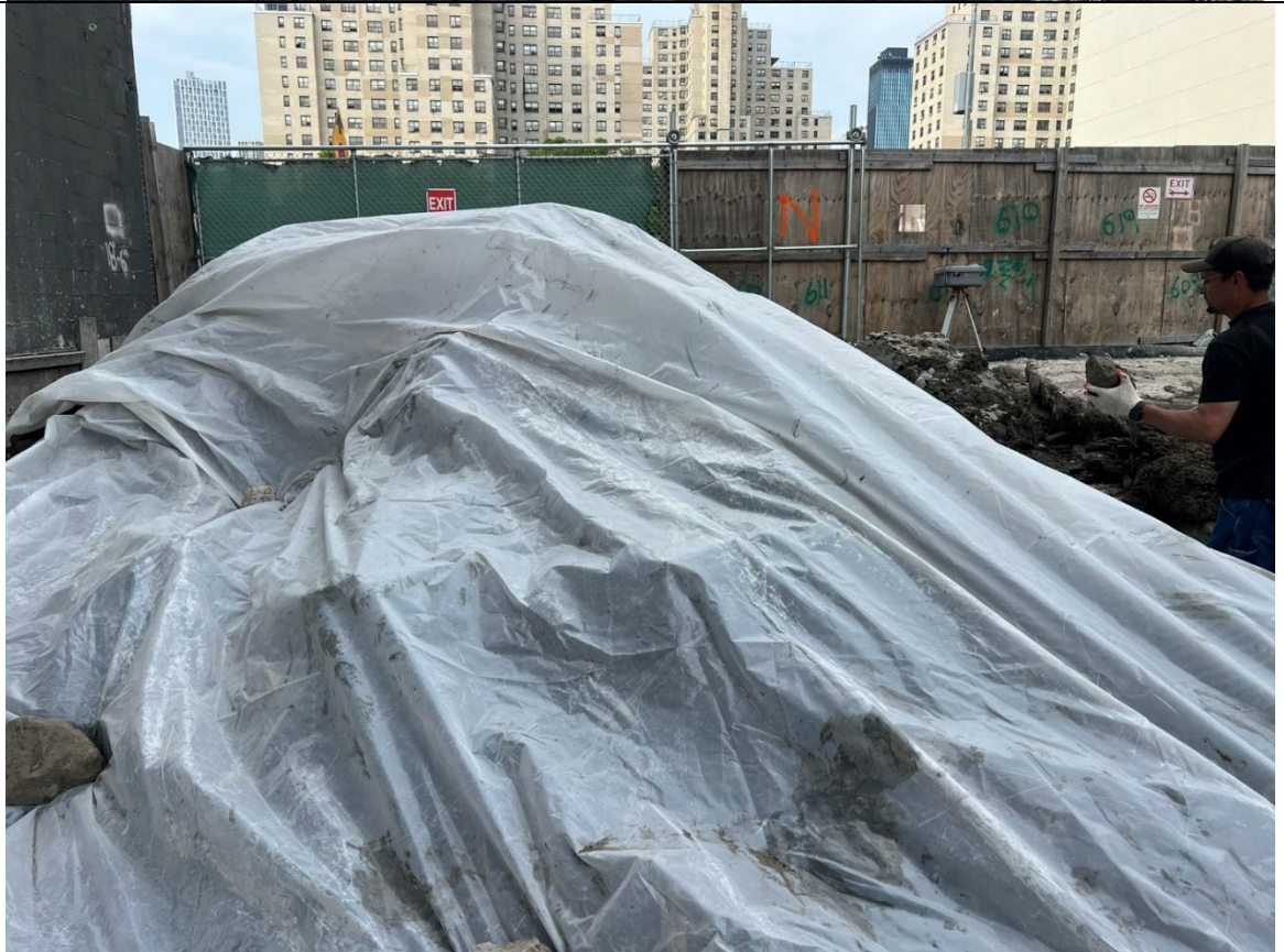
Photo 4- Representative photo of swell stockpile covered with poly at the end of the workday.
