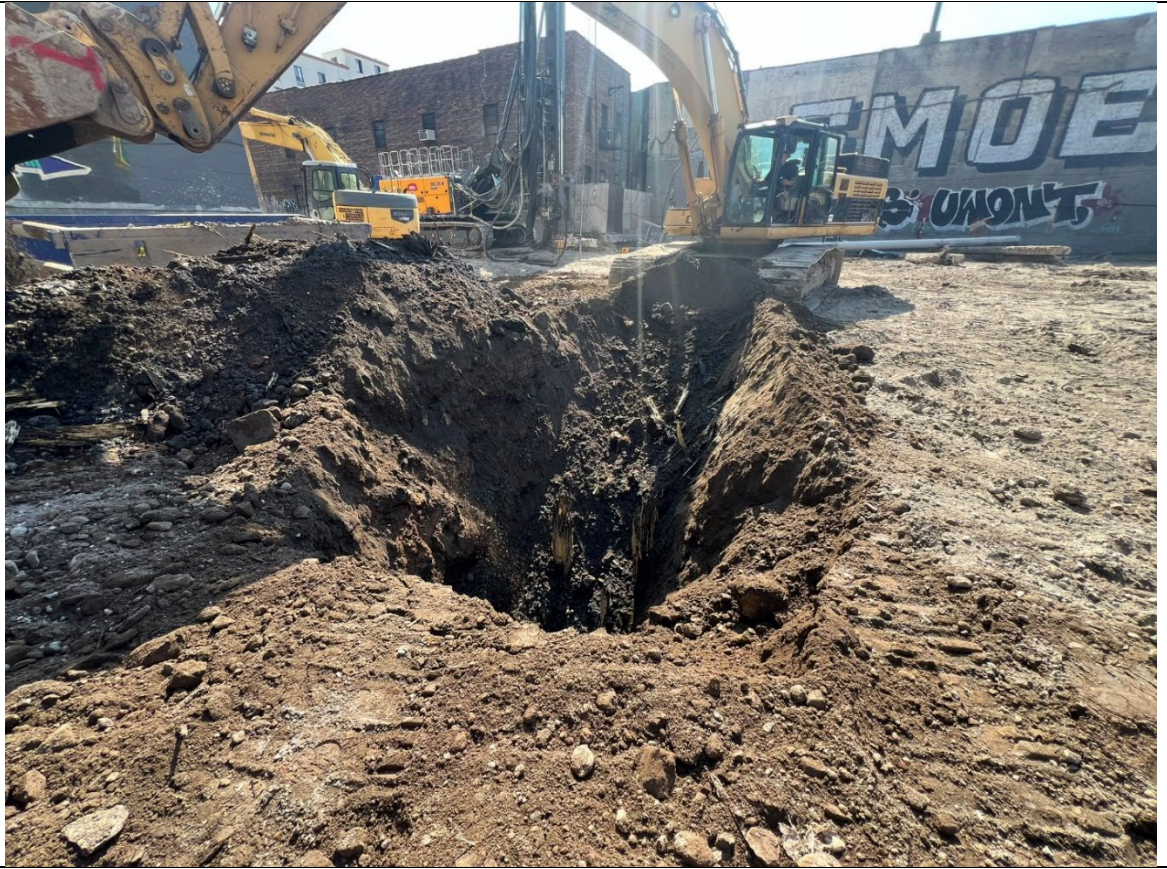
Photo 5- Representative photo of wood piles/obstructions that Concrete Cours removed to the best of their ability.
