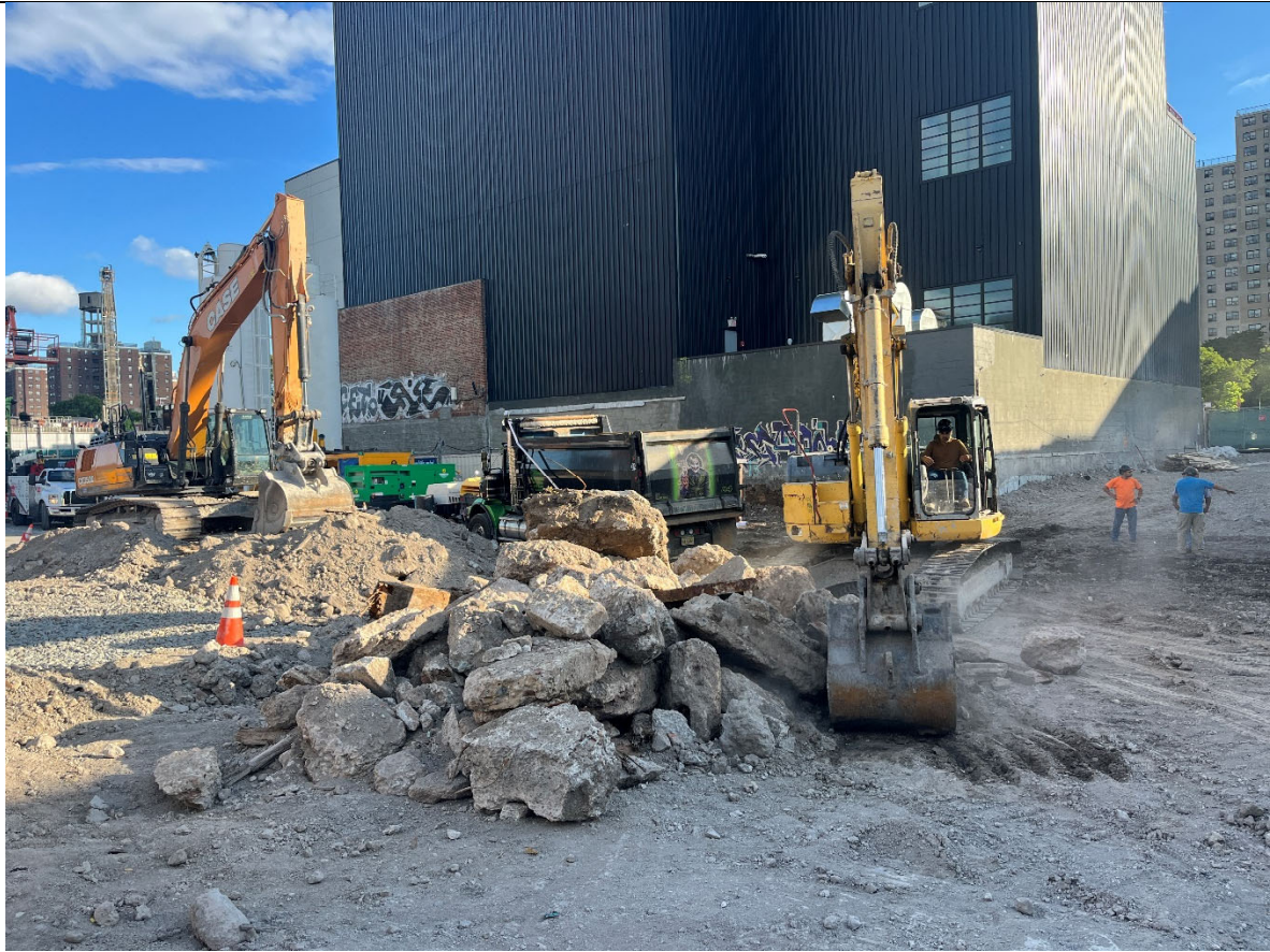
Photo 1- Representative photo of concrete material being removed for offsite disposal to P Park.
