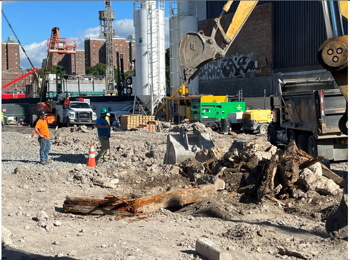
Photo 2- Representative photo of water being utilized for dust suppression during concrete loadout.
