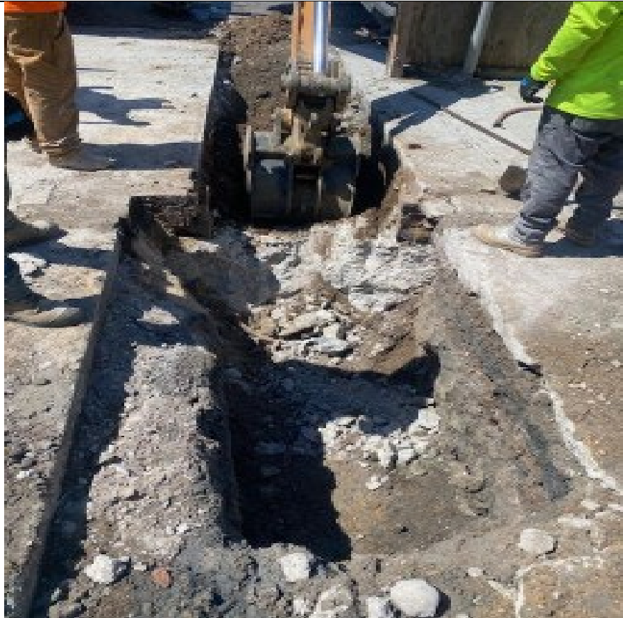
Photo 5- Representative photo of Empire crew excavating within site for sewer connection installation work.
