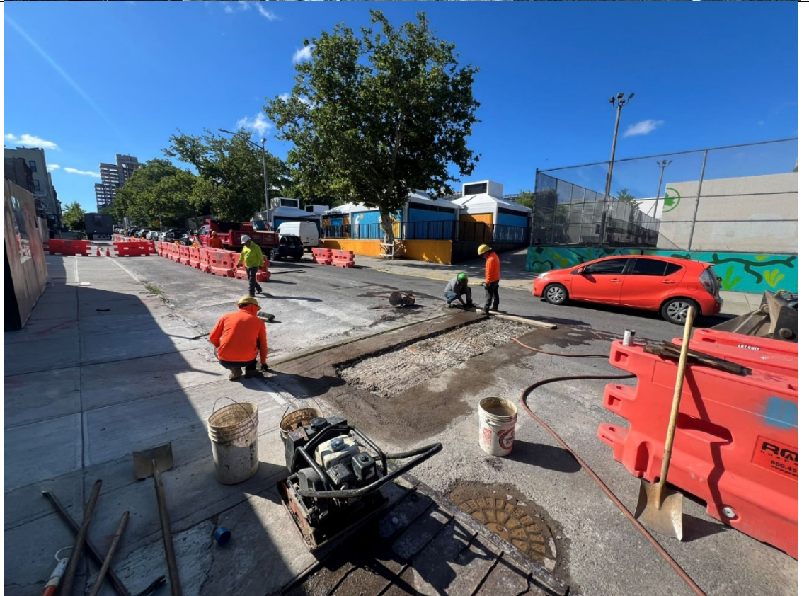
Photo 2- Representative photo Empire repairing the asphalt after the completion of the sewer connection.
