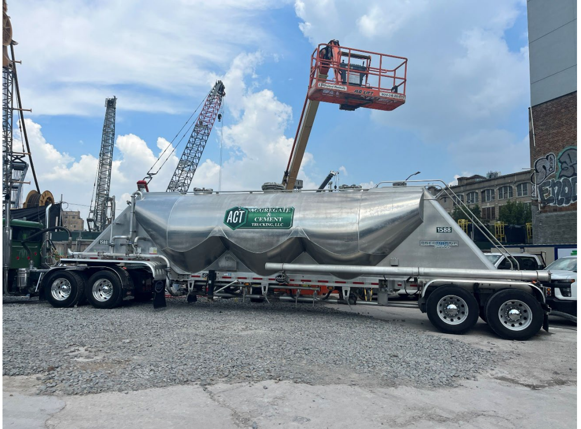
Photo 4- Representative photo of slag delivery to the silo.
