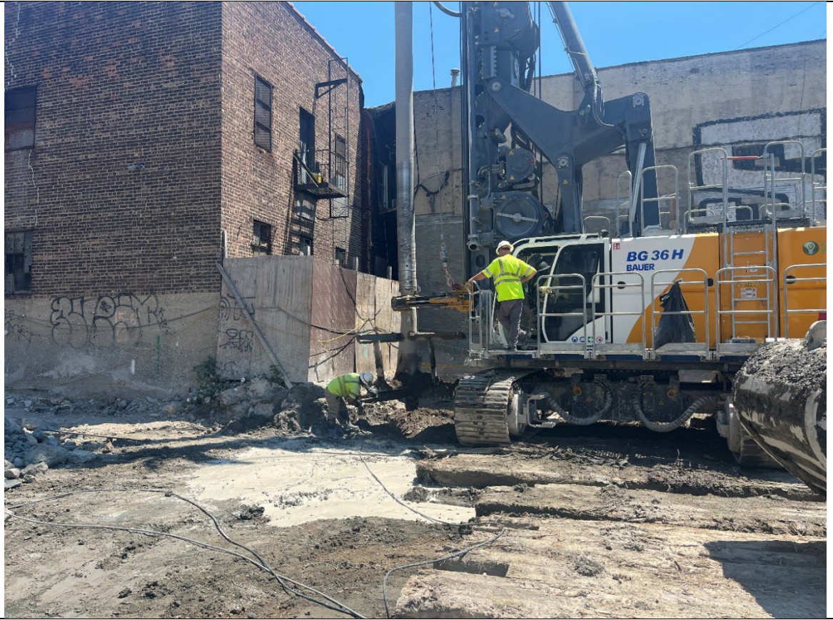
Photo 5- Representative photo of Cascade unclogging grout line and auger for ISS column installation.
