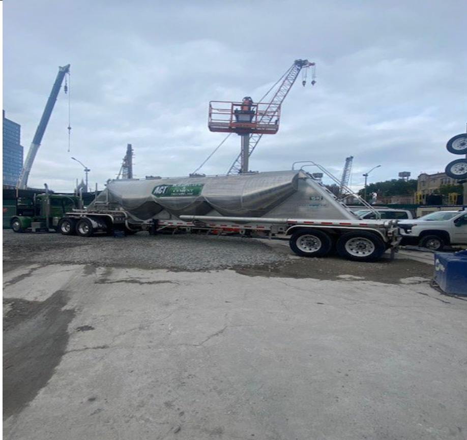
Photo 3- Representative photo of slag delivery to silo.
