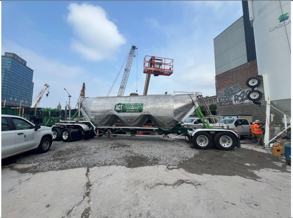
Photo 3- Representative photo of slag delivery to silo.
