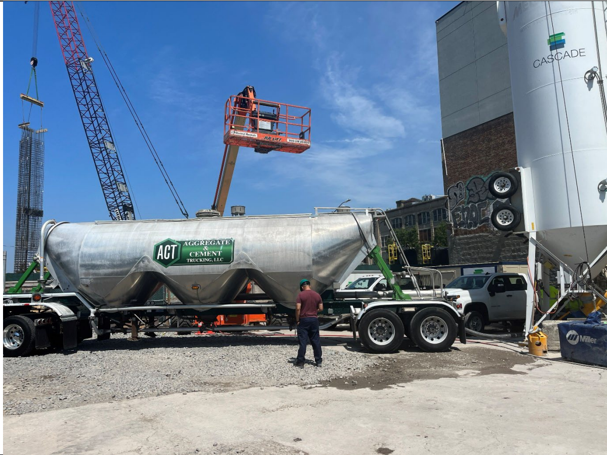
Photo 3- Representative photo of slag delivery to silo.
