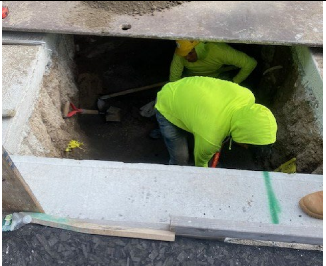
Photo 5- Representative photo of Empire excavating along Butler St. for sewer connection installation.
