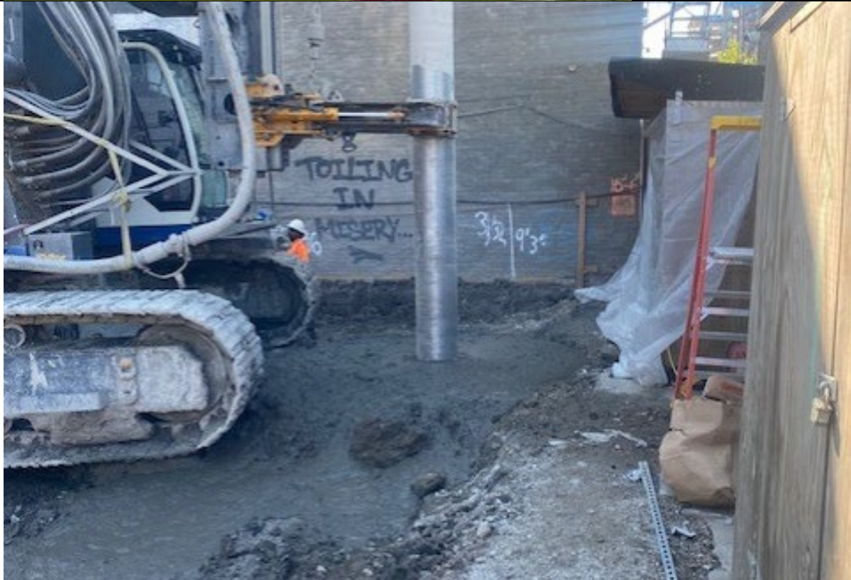
Photo 2- Representative photo of ISS column installation at the southeast corner of the site.
