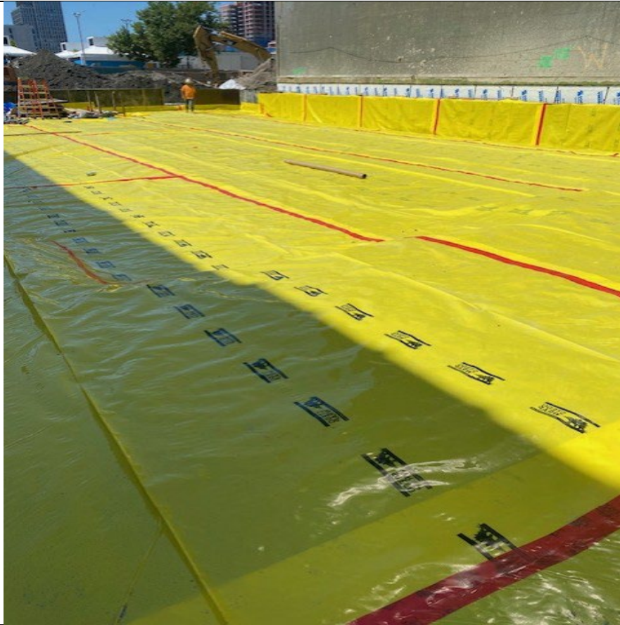
Photo 1- Representative photo of completed vapor-barrier and lumber-form installation in the Butler corridor.
