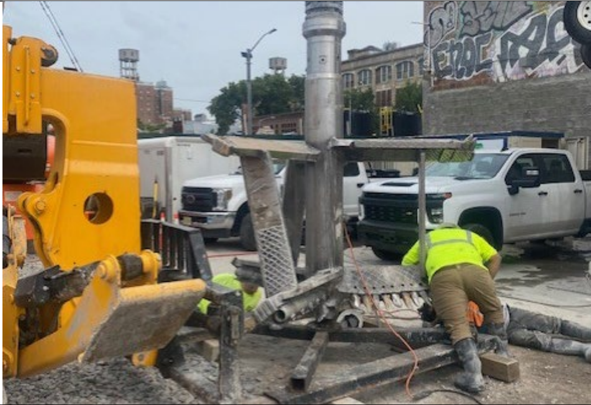
Photo 3- Representative photo of welding and repairs being performed to the ISS auger.
