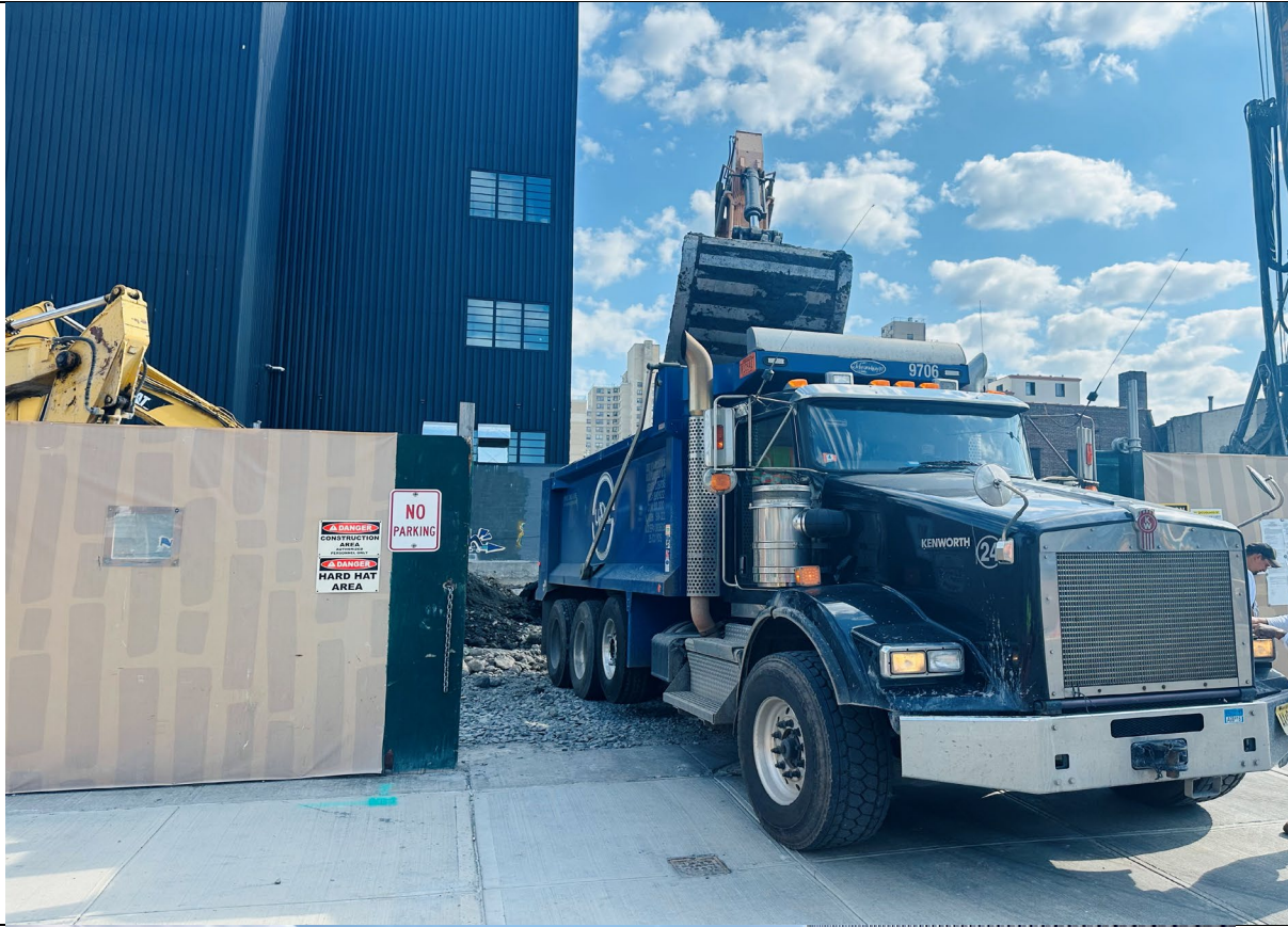
Photo 3- Representative photo of trucks being loaded with swell material to Bayshore facility.
