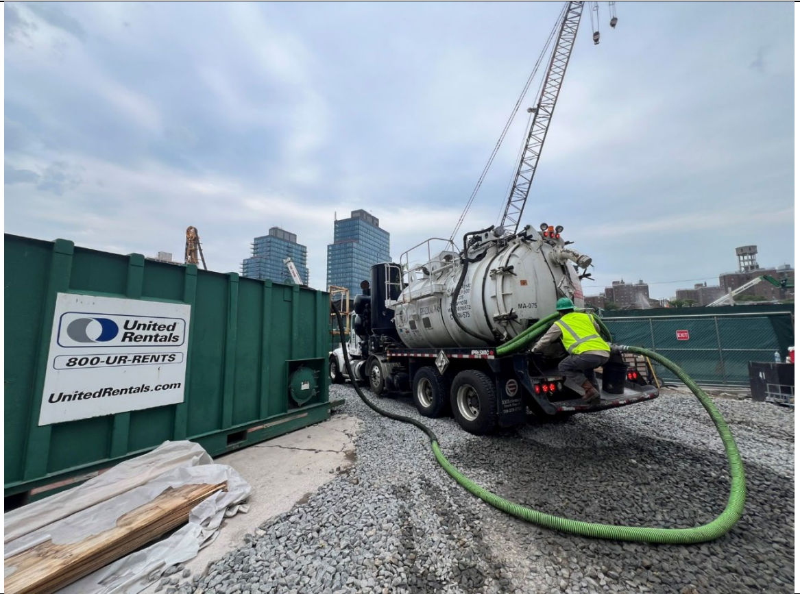
Photo 1- Representative photo of frack tank being pumped out.
