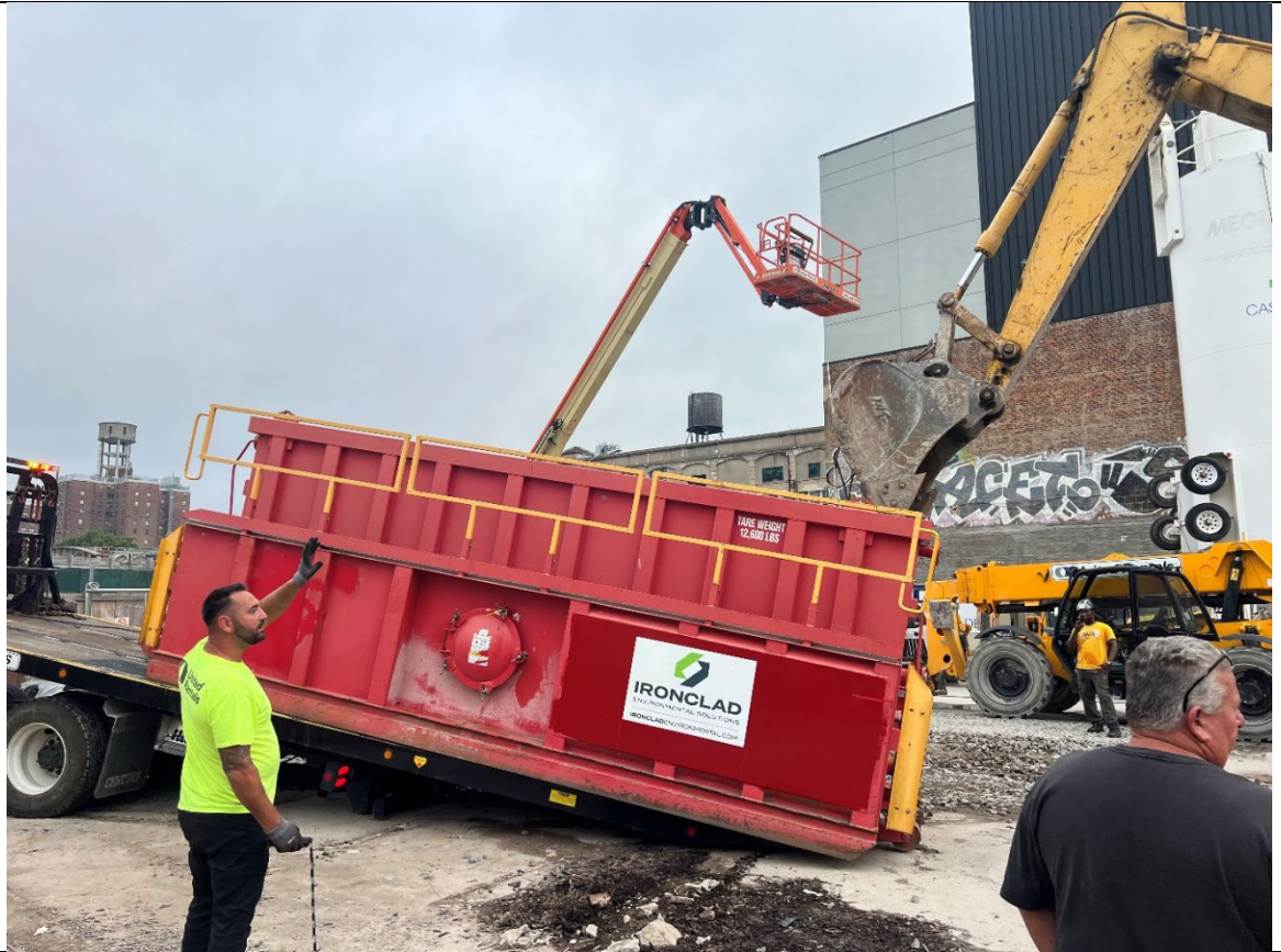
Photo 1- Representative photo of new frac tank delivery.
