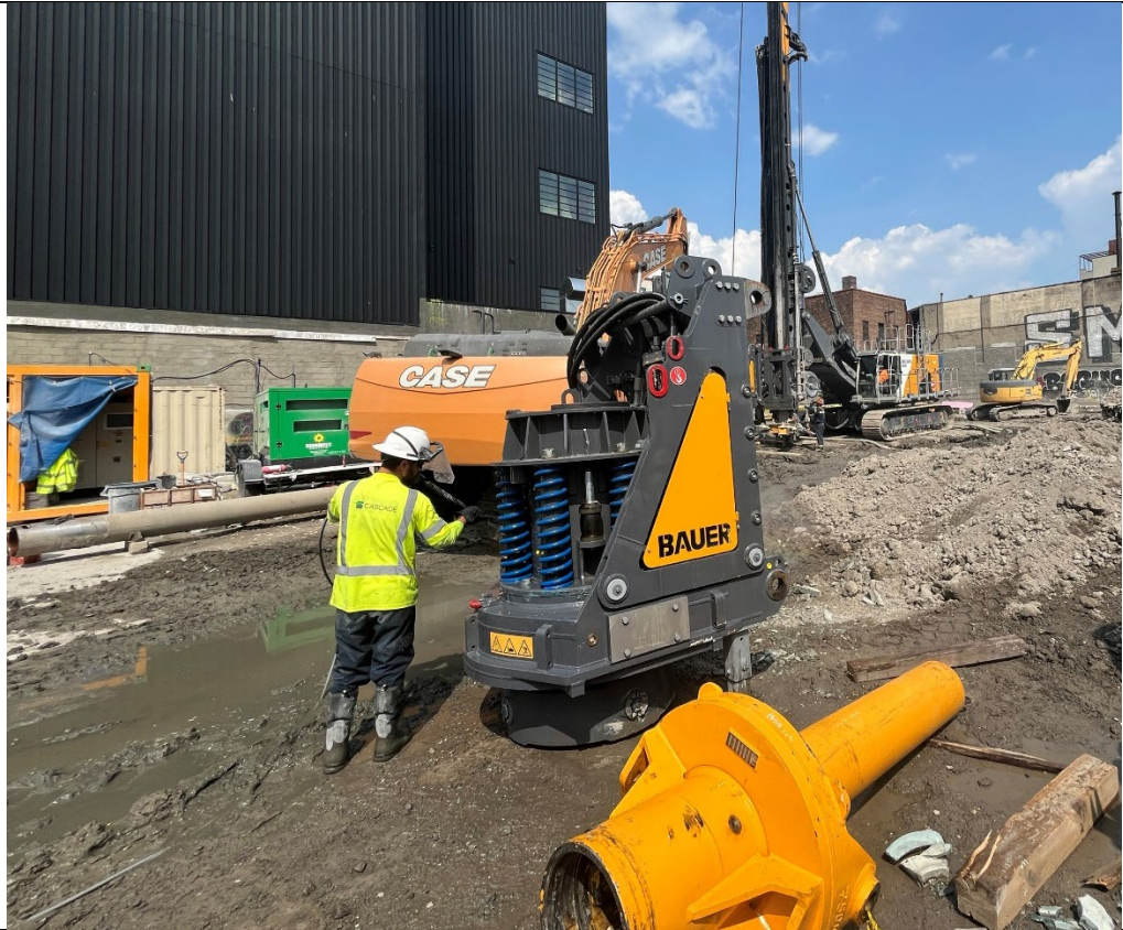
Photo 3- Representative photo of the Bauer KDK removed from the ISS Drill Rig.
