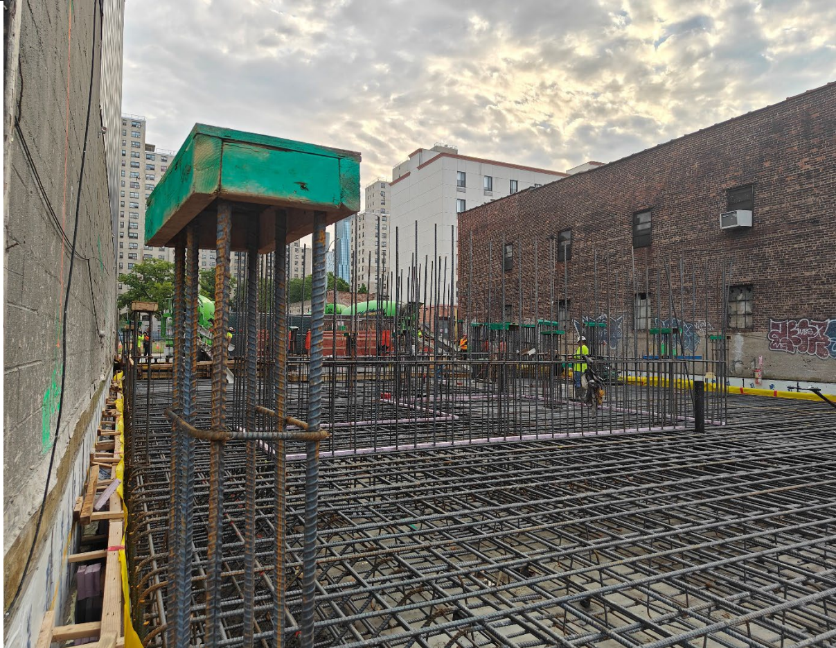
Photo 3- Representative photo of pour area and concrete trucks pouring from Bulter Street.
