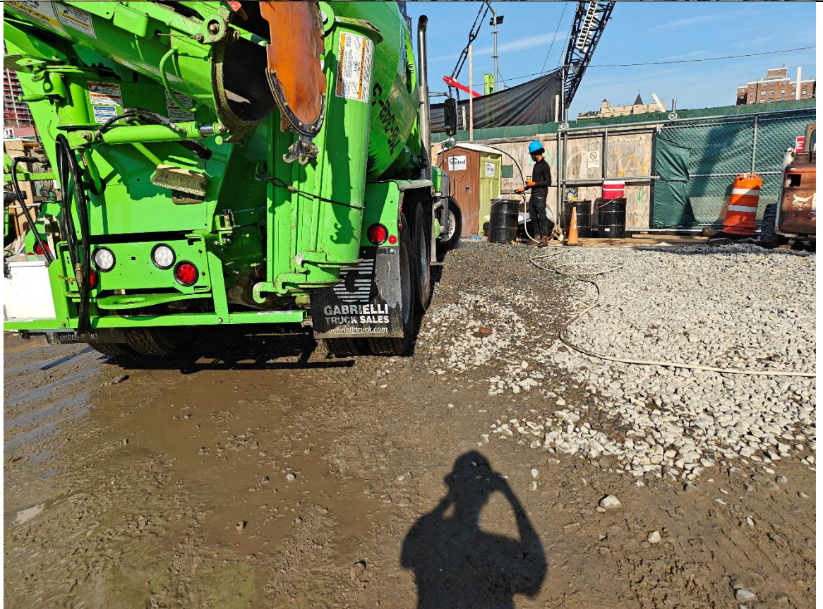
Photo 4- Representative photo of tire washing over track pad prior to trucks leaving the Site.
