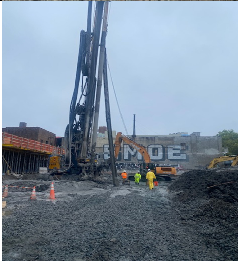
Photo 4- Representative photo of Cascade utilizing bar to collect a wet-mix sample from a completed column.
