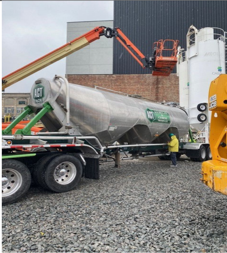
Photo 1- Representative photo of ACT delivering a load of Portland to the silo.
