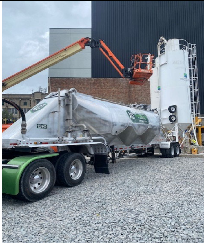
Photo 1- Representative photo of ACT delivering a load of slag to the silo.
