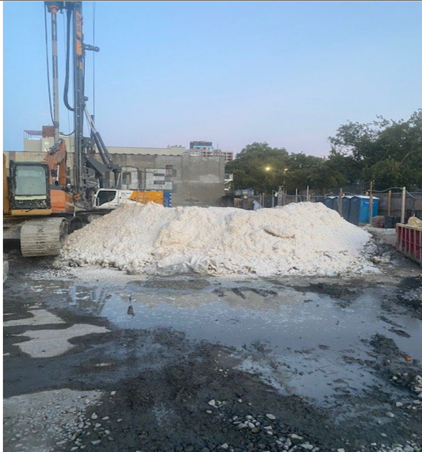
Photo 3- Representative photo of remaining consolidated swell material stockpile applied with ISS spray- foam.
