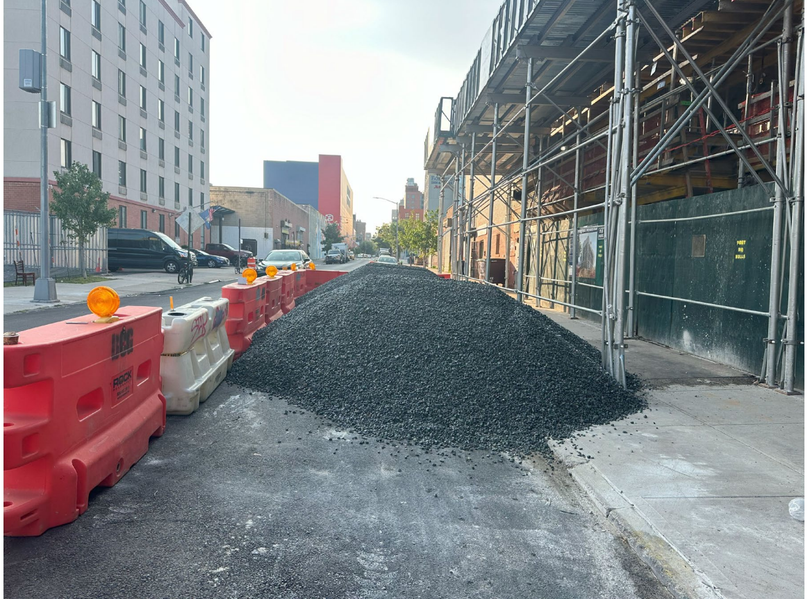
Photo 2- . Representative photo of gravel dumped at Buttler St
