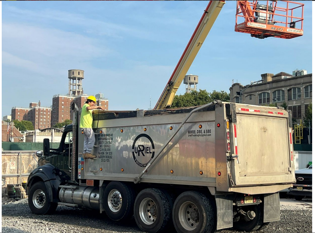
Photo 2- Representative photo of straps being put on the side of a truck prior to exiting the Site.
