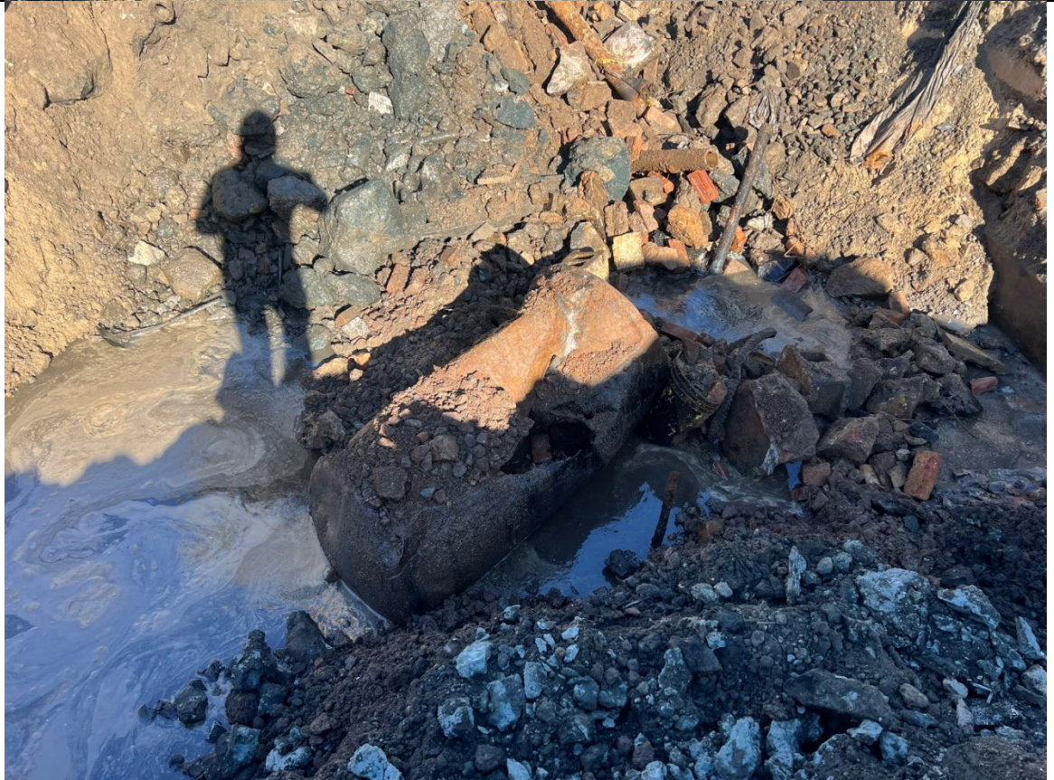
Photo 4- Representative photo of Tank 4 in place.
