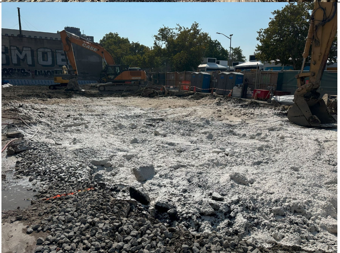
Photo 4 - Representative photo of excavated area sprayed with foam at the end of the day.
