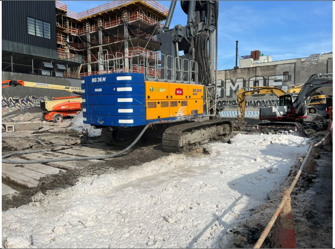
Photo 5- Representative photo of work area covered with ATMOS foam at the end of the day.
