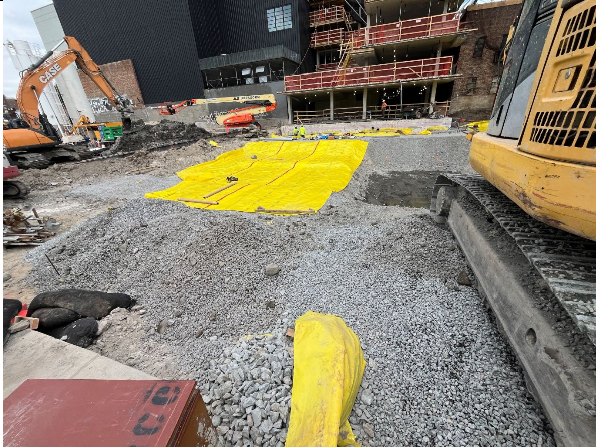
Photo 2- Representative photo of vapor barrier installation in progress in the eastern portion of the Site.
