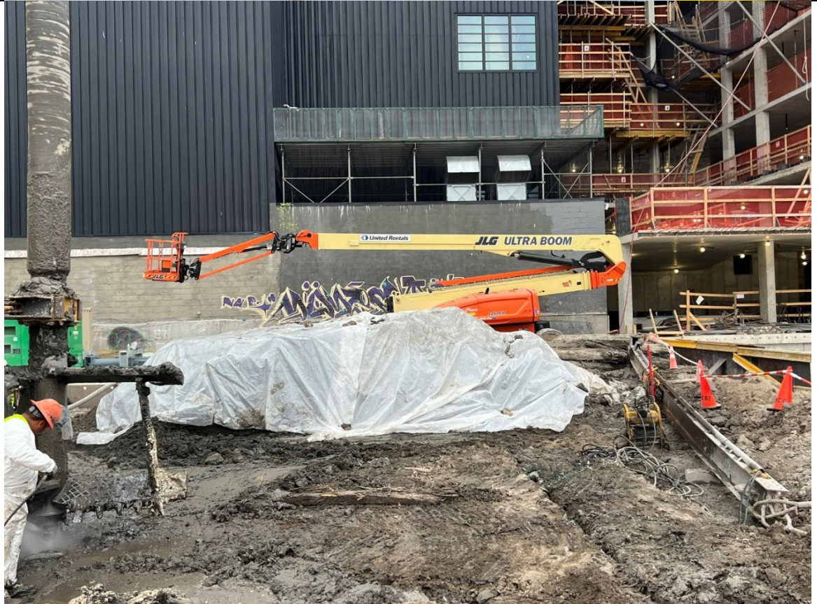
Photo 4- Representative photo of swell stockpile covered with poly at the end of the day.
