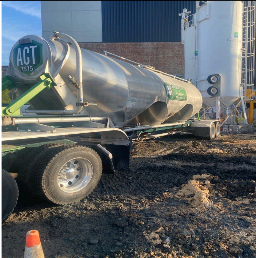
Photo 1- Representative photo of slag delivery to the silo.
