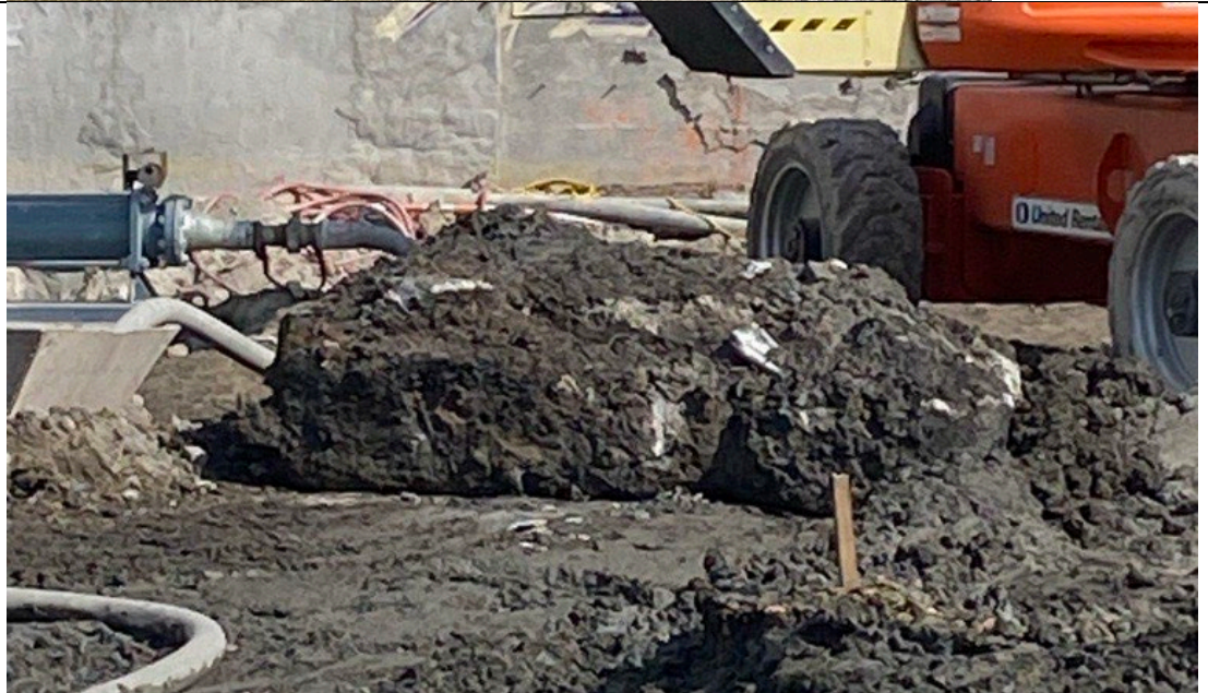
Photo 4- Representative photo of large section of concrete foundation excavated from area of column installation.
